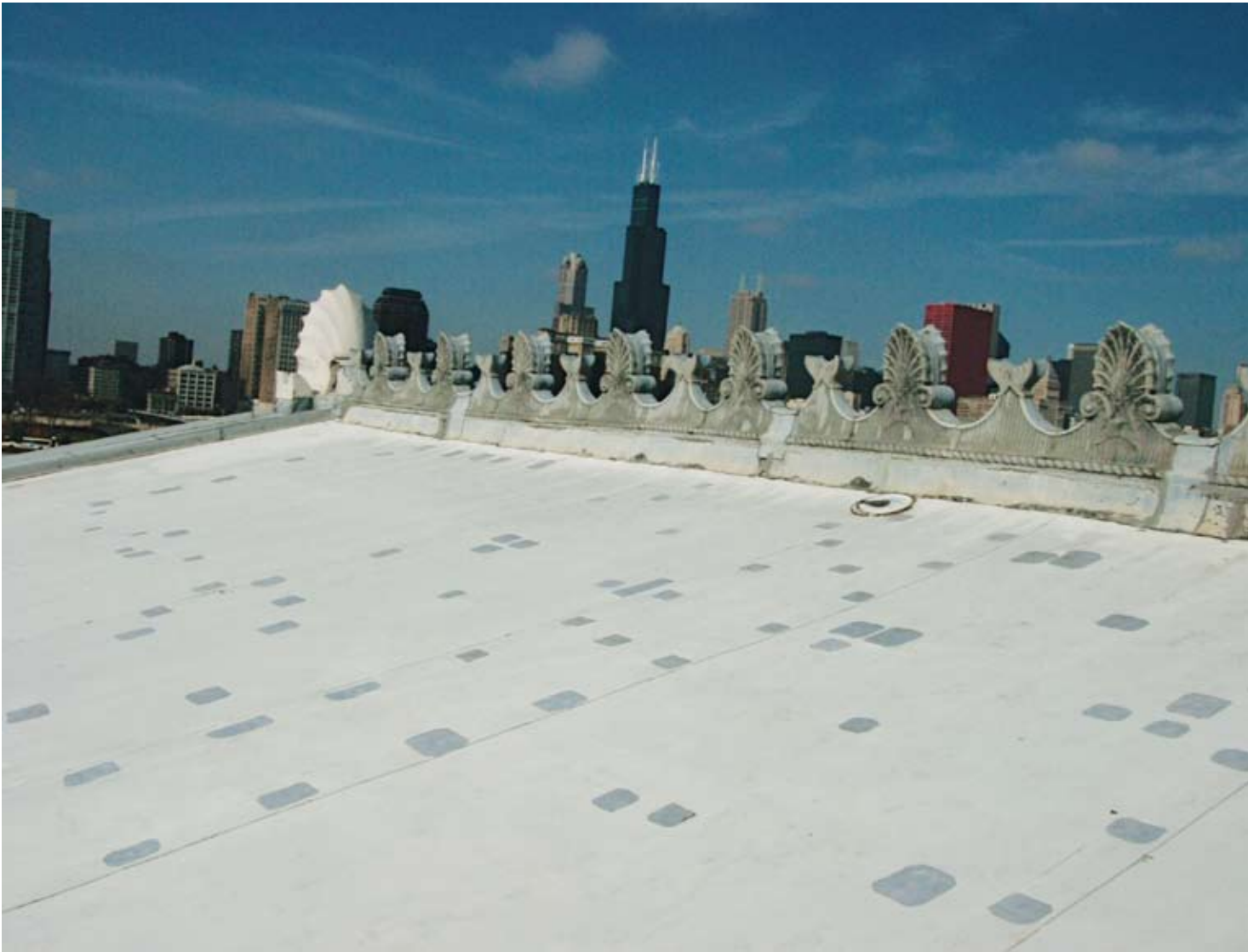
■ EternaBond was used to patch holes in the roof at the John G. Shedd Aquarium in Chicago before a soy oil polymer-based roofing system was applied. (Photo courtesy of EternaBond.)
