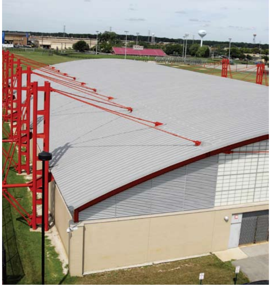
■ Approximately 30,000 linear feet of RoofSeal was used to repair the seams on the metal roof at the Niles West High School field house in Skokie, Ill. (Photo courtesy of EternaBond.)
