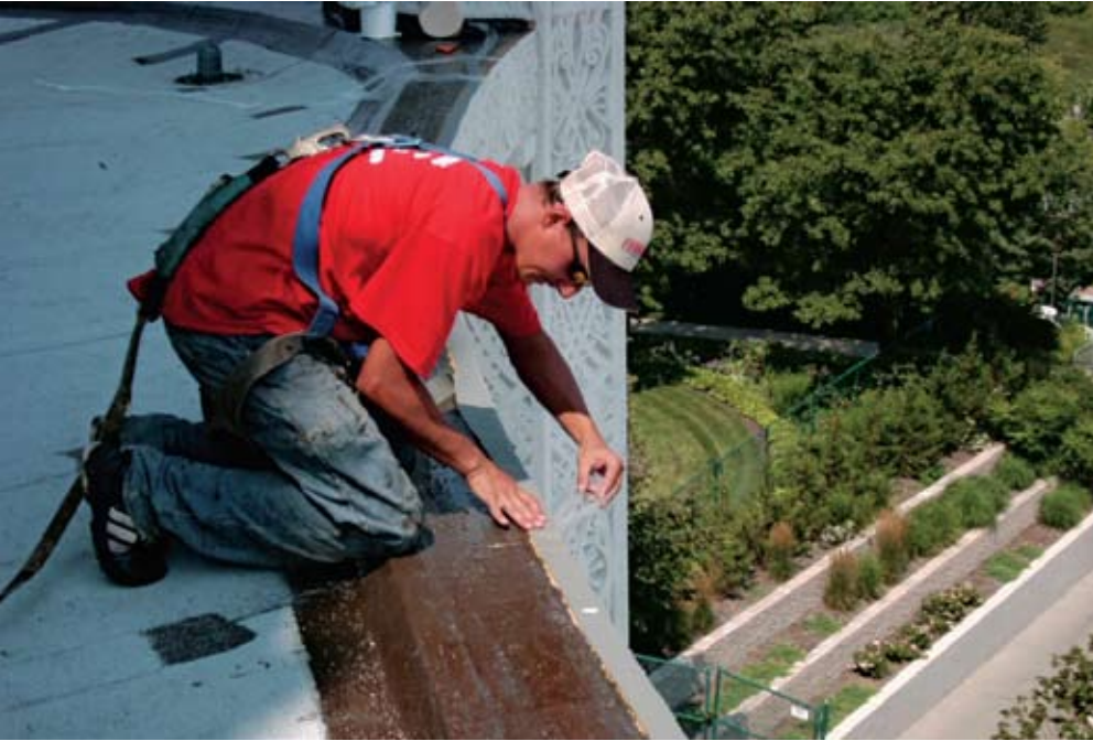
■ At the Shedd Aquarium project, EternaBond was used to repair roof leaks, as well as securing copings and flashings.
